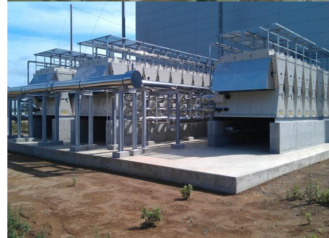
Chiller system for Helios (JA procurement)
